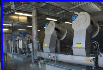
8 Solids Handling: Stabilize and reduce the amount of water in remaining in the solids.
