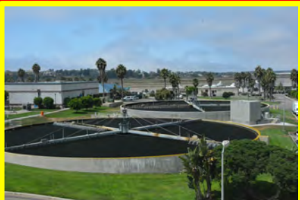
Step 3 Biofilters: Convert soluble contaminants to suspended and settleable solids.
