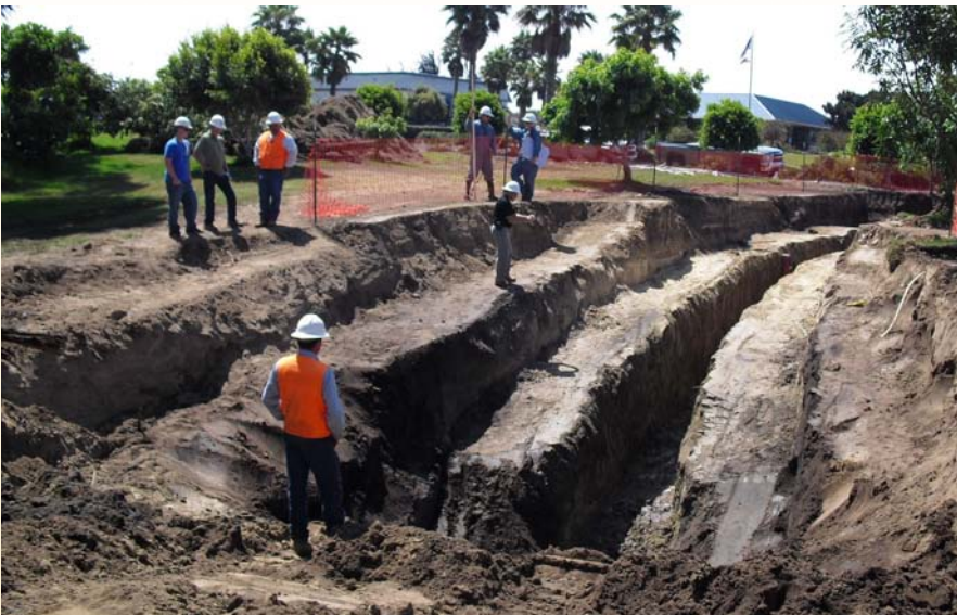
Trench for the earthquake fault study conducted prior to the treatment plant upgrade project.
