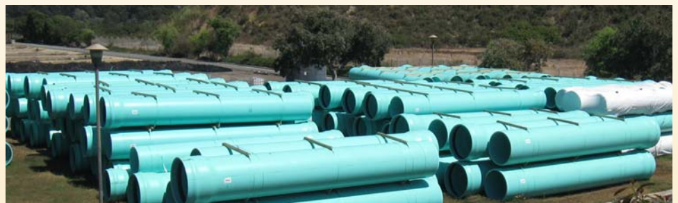
The new sewer pipeline will replace an aging pipeline along San Pedro Creek.
