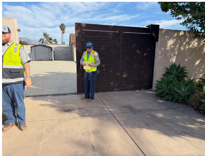
Photo 2: Station locked entrance gate; operators estimate flows of approx. 150K to 200K gallons per day through station
