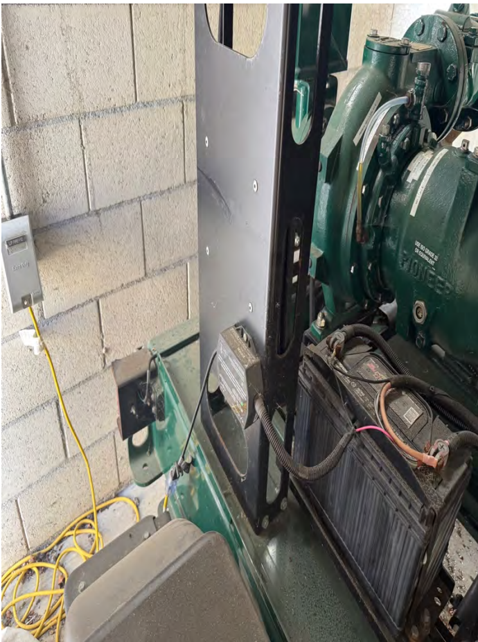
Photo 7: Inspection (station generator on battery tender for emergency readiness)
