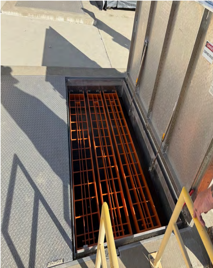
Photo 21: Inspection (force main valve pit); no scheduled valve exercising program (only periodic/intermittent valve exercising practices)
