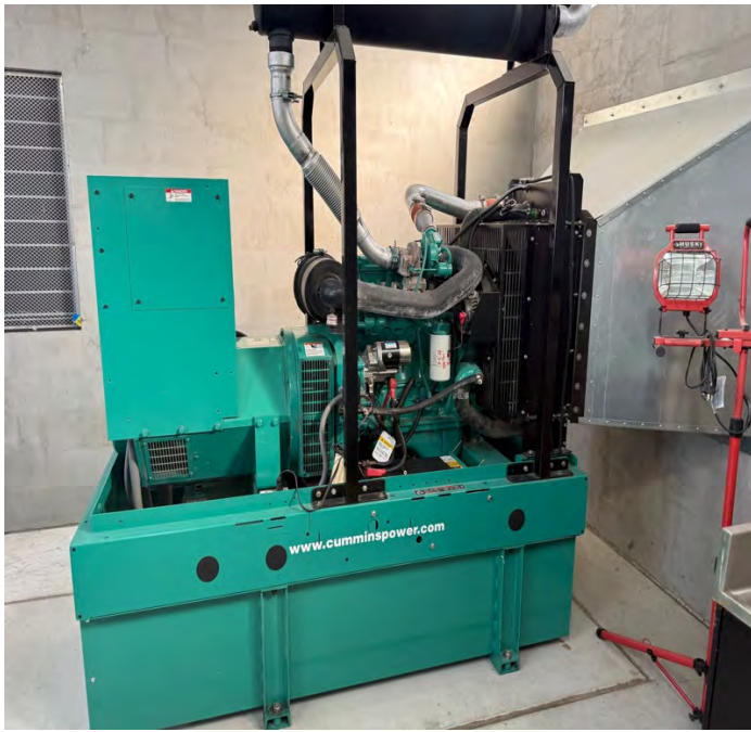
Photo 9: Inspection (station dedicated onsite generator)
