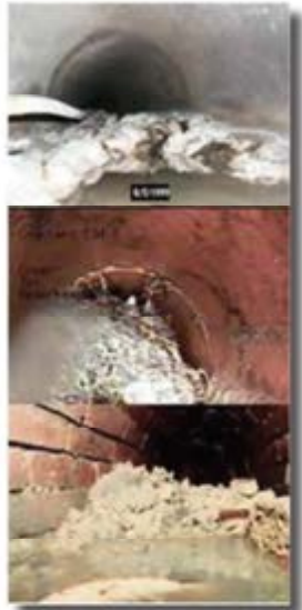
Examples of Service Defects in a Pipe
